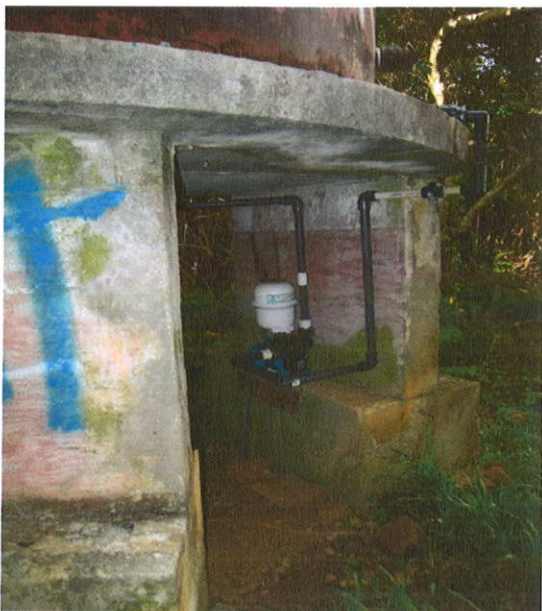
11/2/15: On-Site Visit: Emmaus High School, 2 of 2 Electrical Water Pumps, installed after September 15, 2015.
