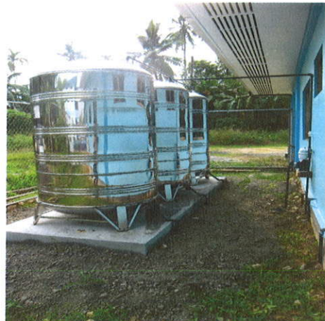
10/19/15: Installed PCAA Water Catchment System, no electrical switch panel; therefore, system is still incomplete.
