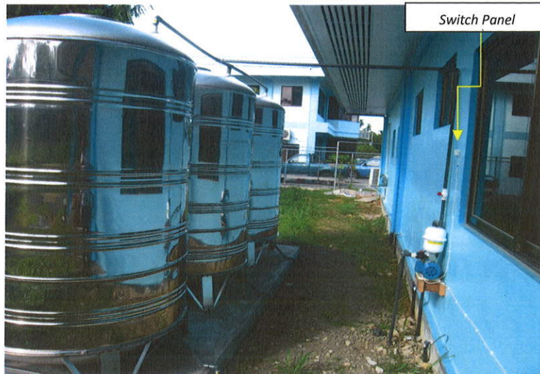
Completion of all works on Water Catchment System for PCAA Head Start Center on 10/29/15.
