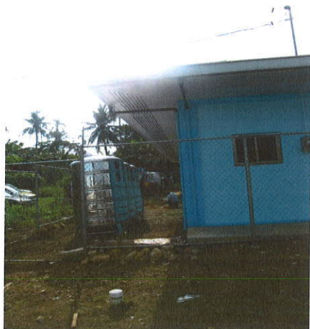
9/28/15: FR Construction Co. employee working on concrete base for the water tanks.
